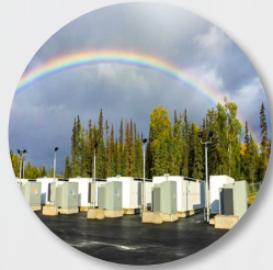
Battery Energy Storage System (BESS) 46.5 MW
