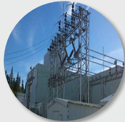
Bernice Lake Combustion Turbine Plant 76.0 MW
